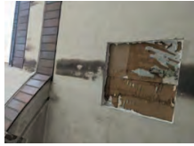
17 EIFS CONDITION AT EXT. MEZZANINE 18' x 12'
