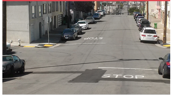
Unacceptable paving restoration
