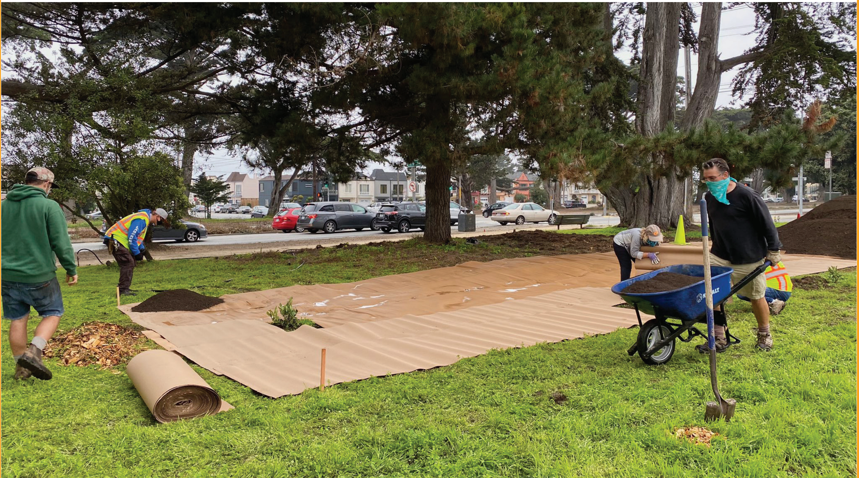
Prior to planting, cardboard is laid down to keep weeds from sprouting.
