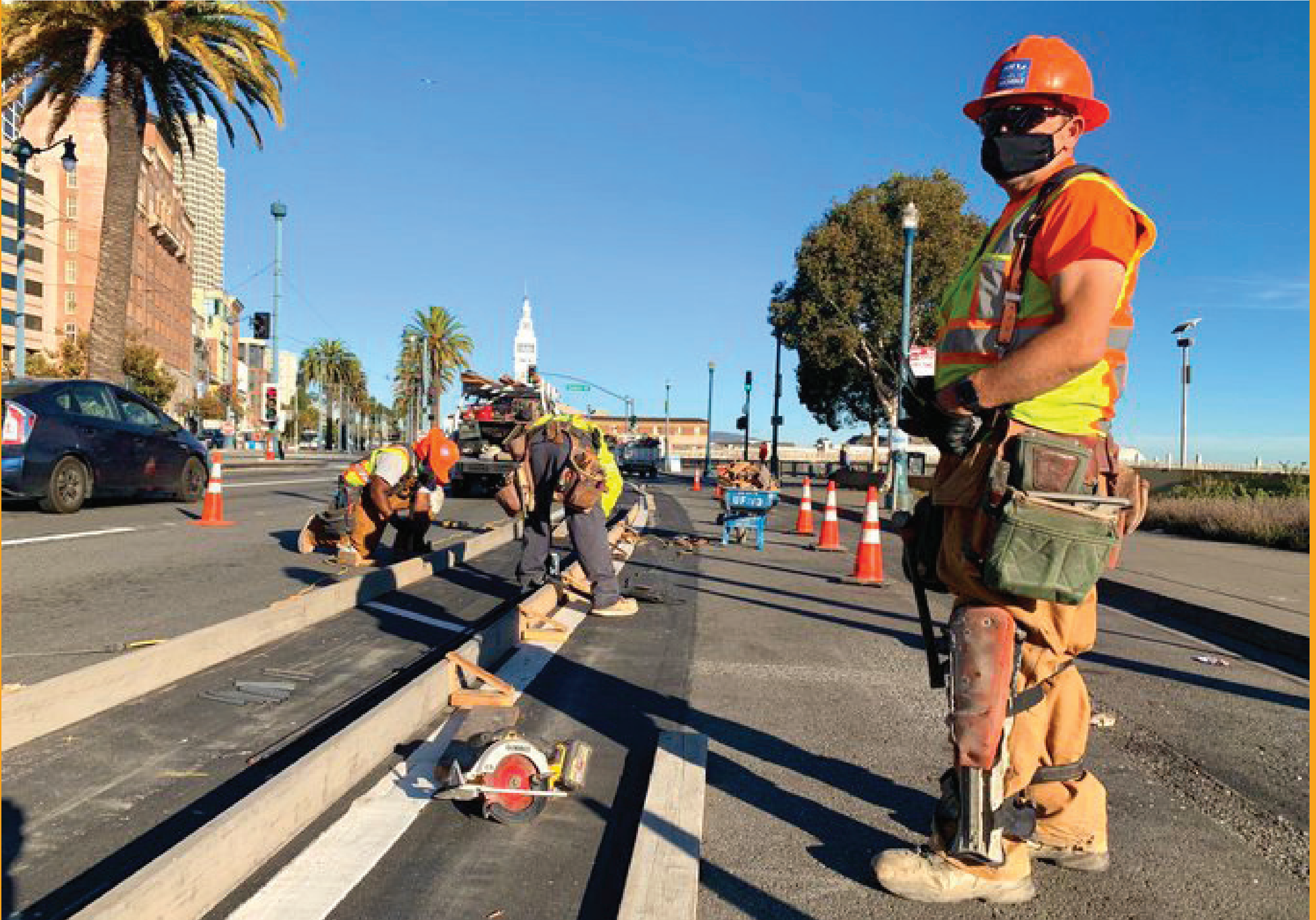
Top left: Public Works Cement Mason Ernesto Munoz smooths out a new island. Top right: A finishing trowel is used to achieve a smooth texture. Bottom: Cement Mason Gabriel Arteaga from our Bureau of Urban Forestry Cement Shop stands watch as crews build the wooden frames to support the freshly poured islands.
