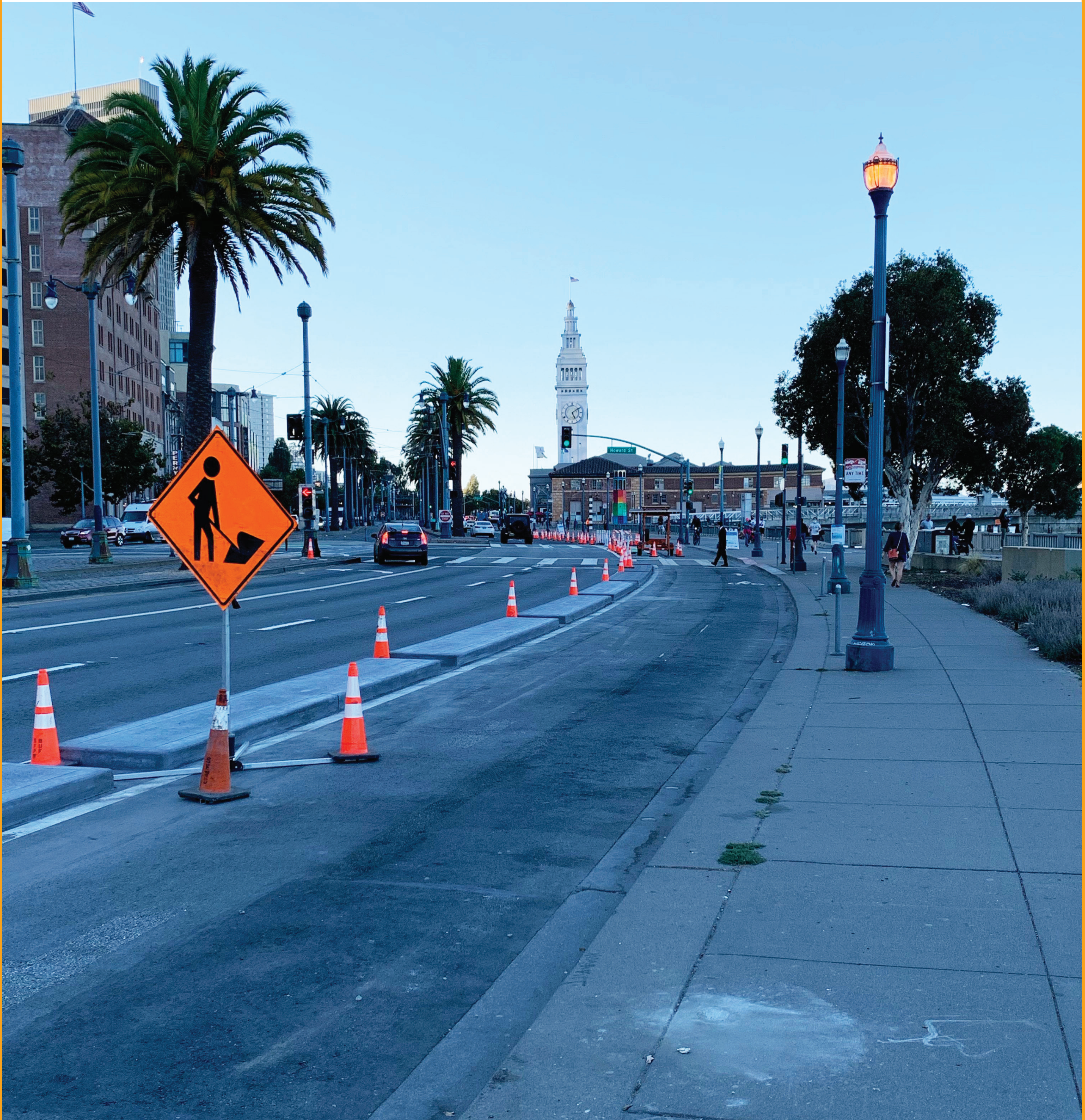
A total of 49 concrete islands, hand-built by Public Works crews, separate bikes from vehicles.
