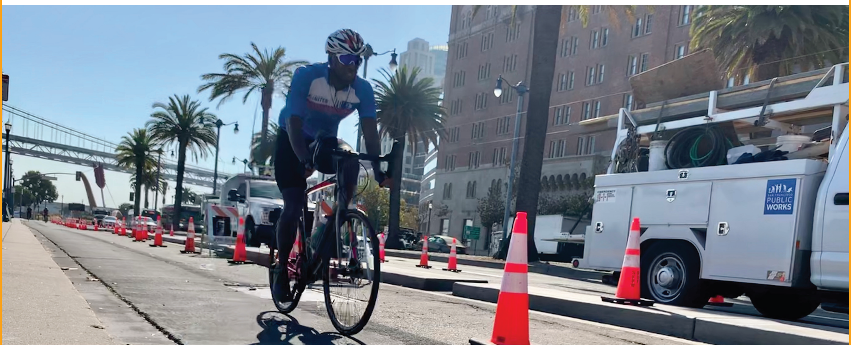
A lone cyclist tests the new protected bikeway before construction is complete.
