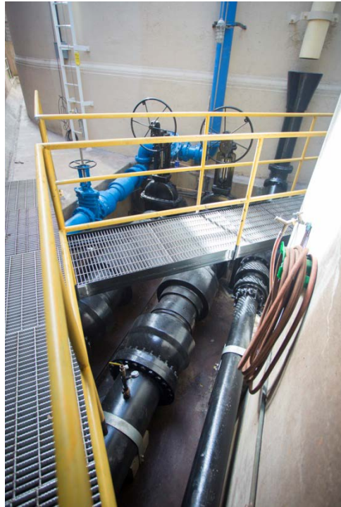
Jones Street Tank, new piping and walkway
