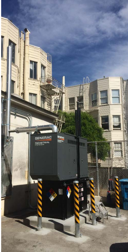
Station 12 – Emergency Generator
