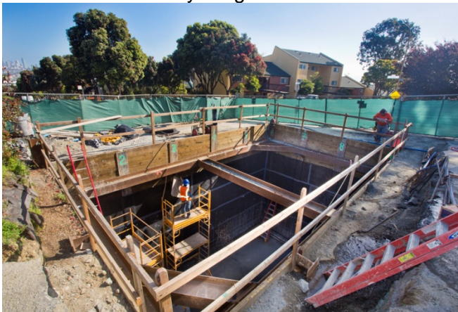
Cisterns at Cashmere St. & Hudson Ave.
