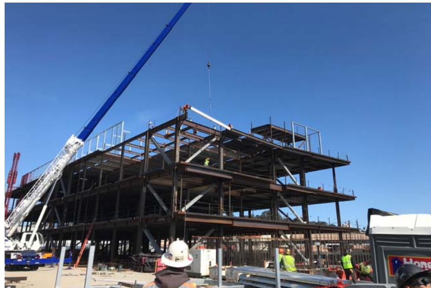
Traffic Company & Forensic Services Division Topping-Out – Erection of Final Steel Beam – April 3, 2020
