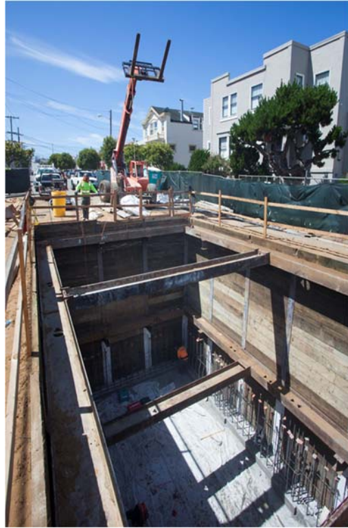
18th Avenue & Moraga Street cistern
