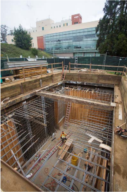
Laguna Honda Hospital cistern
