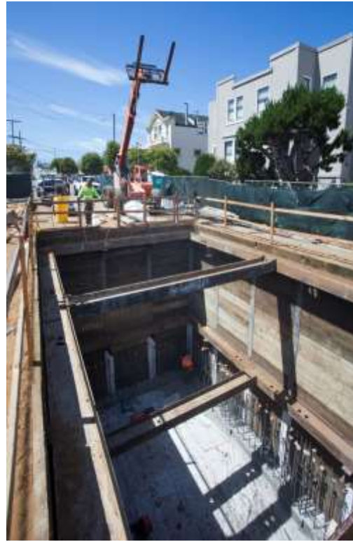
18th Avenue & Moraga Street cistern
