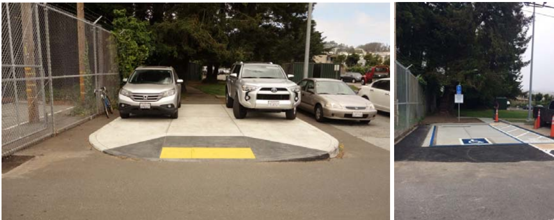
Ingleside Police Station – Before and after photos of new accessible parking space and signage.
