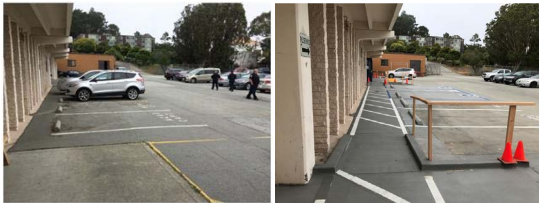
Police Academy – Before and after photos of new accessible parking space and path of travel
