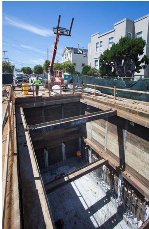
18th Avenue & Moraga Street cistern
