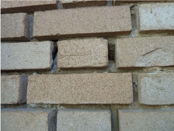
Existing brick pointing failing
