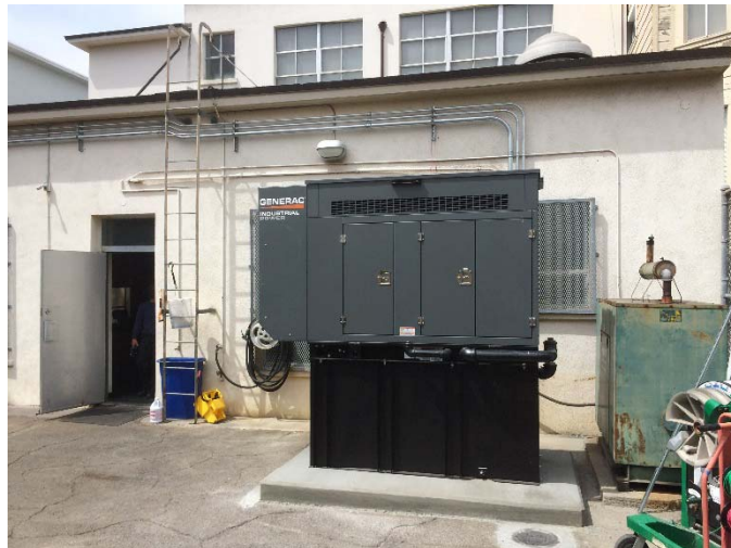
FS21 emergency generator
