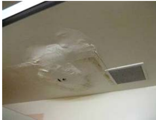
Ceiling damage at fire station
