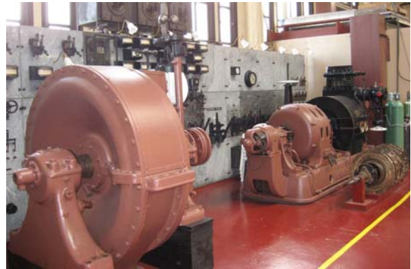
Steam Turbines Electric Generator
