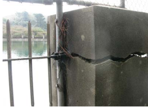
Cracked reservoir pilaster
