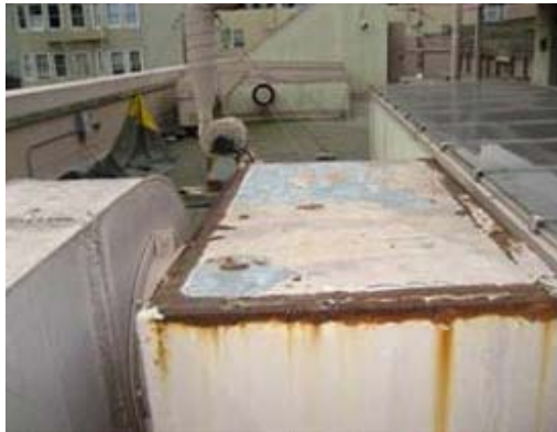
Damage of mechanical equipment at fire station
