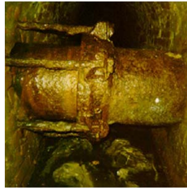
AWSS corroded pipe
