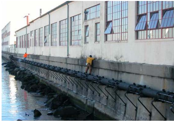
AWSS pipes along sea wall to bayside fireboat
