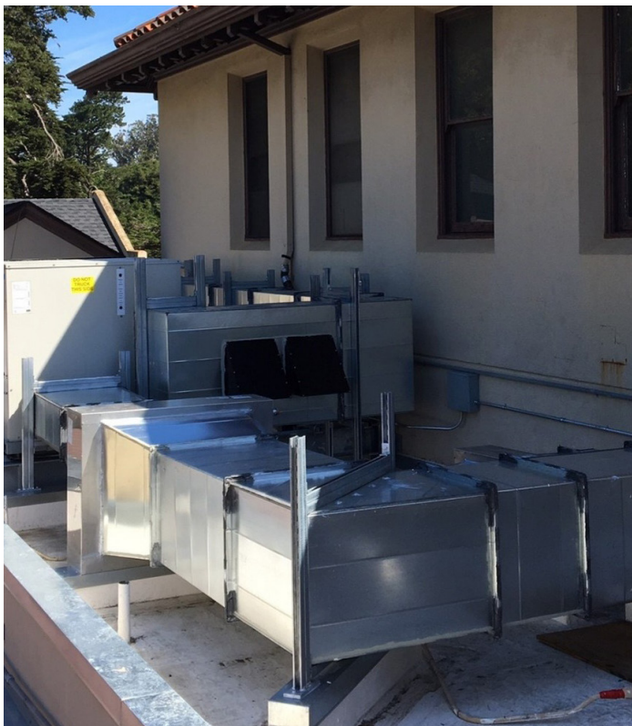
New HVAC unit at Park Station
