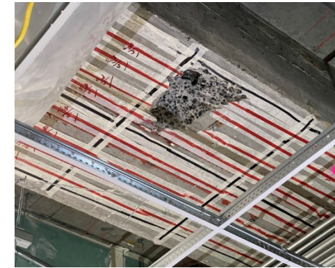
Example of PT Damage
