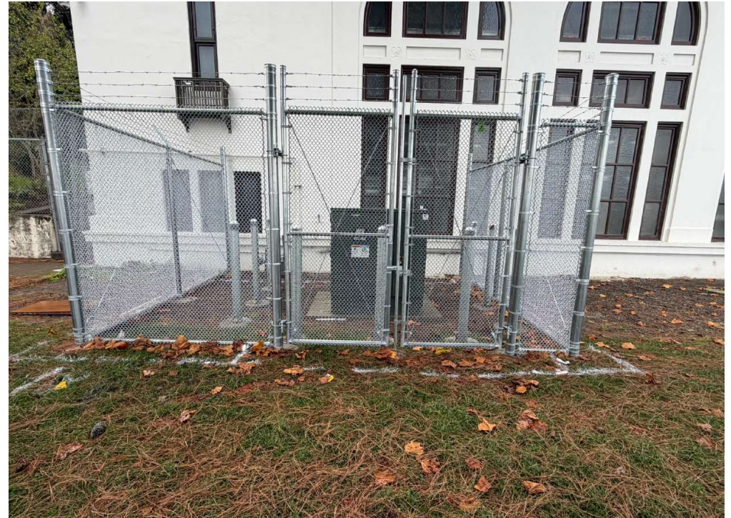
Pumping Station No.2 – Installed electrical equipment
