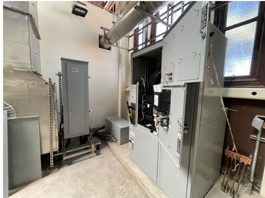
Pumping Station 2 at Fort Mason
