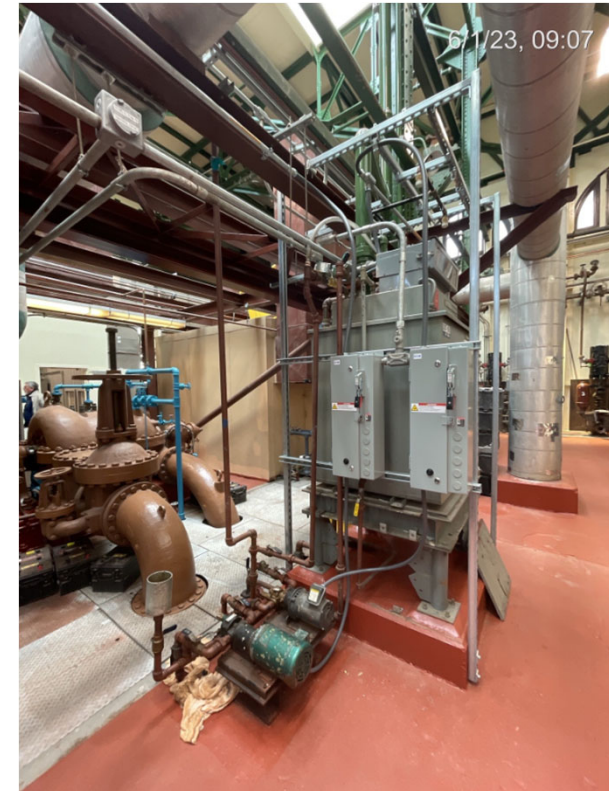
Pumping Station 2 at Fort Mason
