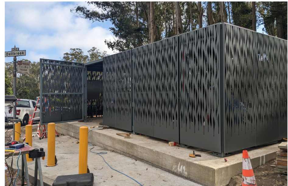
Clarendon Supply project: Enclosure installed
