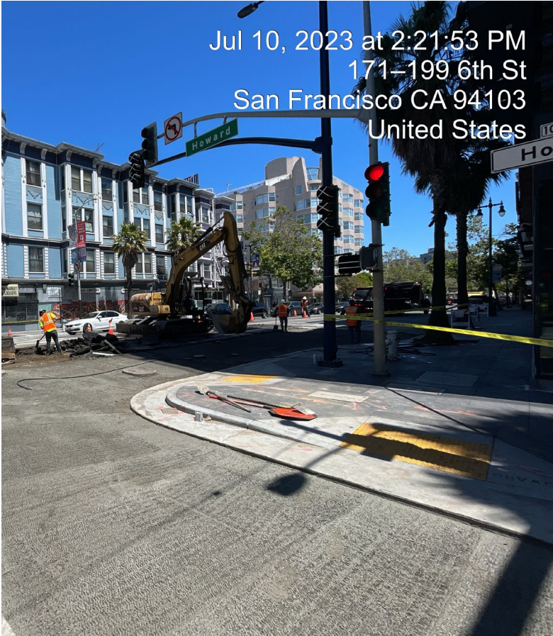
6 th and Howard, New traffic signals
