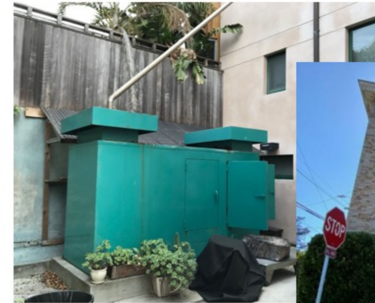
FIRE STATION 37 798 Wisconsin St
