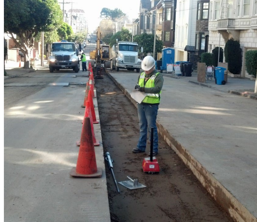
ASTM D6938 In-Place Density test performed on field site for compacted subsurface soils.
