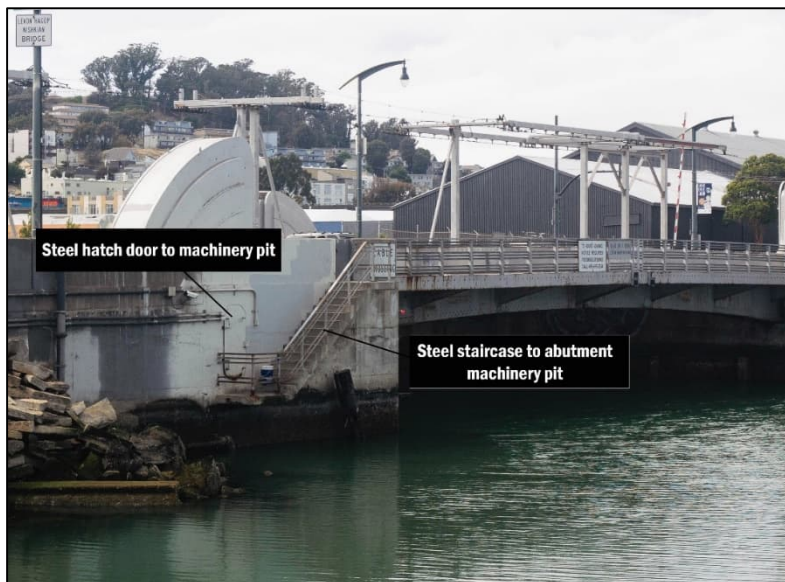
Photograph 3. Character-Defining Steel Staircase Leading to Abutment Machinery Pit, and Sidewalls of Concrete Abutments at Southeastern Corner Leading to Steel Hatch Door, Facing Northwest
