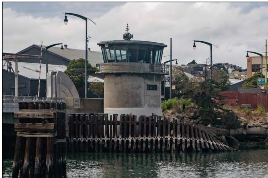
Photograph 8: Two-story, oblong-plan concrete control tower at the northeast corner of the bridge with fender pile system at base in waterway at base of tower, facing northwest
