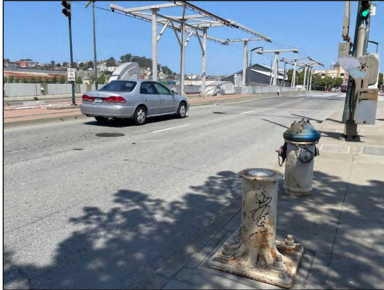
Photograph 10: AWSS hydrant with blue bonnet at southeast corner of Islais Creek Bridge, facing north
