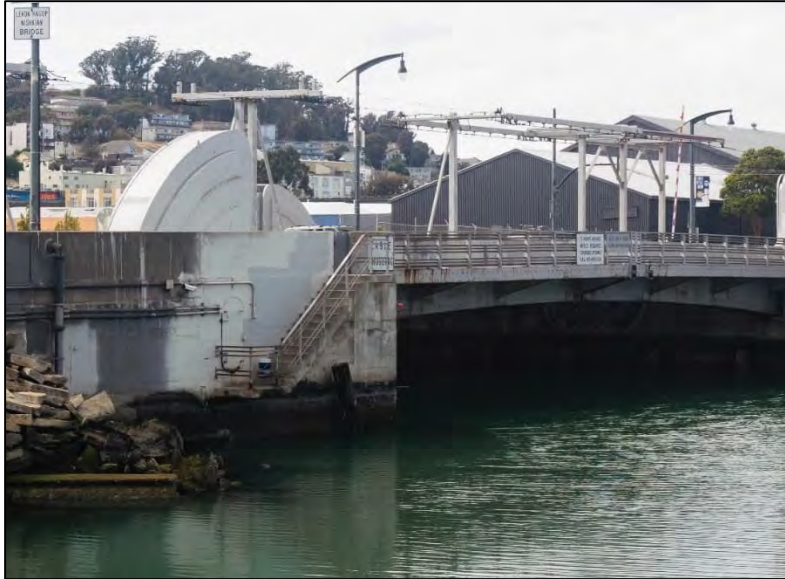
Photograph 5: Sidewalls of concrete abutments and machinery pit, showing stairs on southeast corner leading to steel hatch, facing northwest
