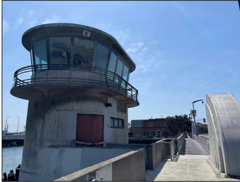
Photograph 9: Control tower with canted window configuration, walkway and handrails surrounding the top floor, copper roofing with overhang, and door and window configuration, facing south
