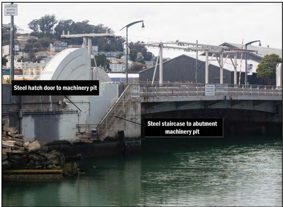
Photograph 3. Character-defining steel staircase leading to abutment machinery pit and sidewalls of concrete abutments at southeast corner leading to steel hatch door, facing northwest
