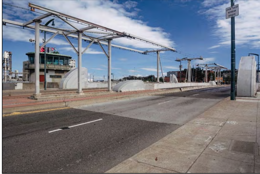
Photograph 3: Two quarter-round and one teardrop-shaped girder housing units with Art Moderne styling near the north end of Islais Creek Bridge, facing southeast
