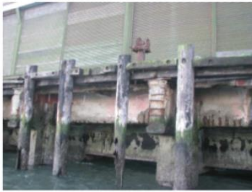
3 EXISTING FENDER SYSTEM TO BE REMOVED. EDGE AND INTERMEDIATE BEAMS TO BE REPAIRED.
