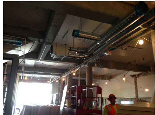
HVAC Duct Work at App Bay Ceiling
