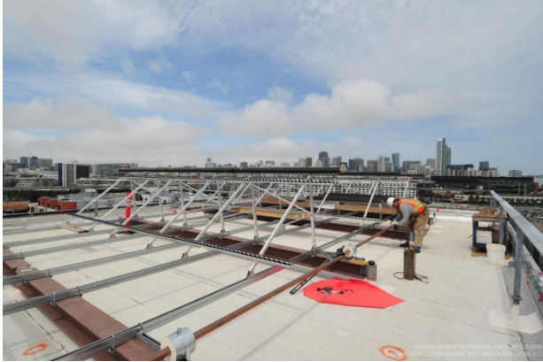
Support for communication rooftop equipment at West tower
