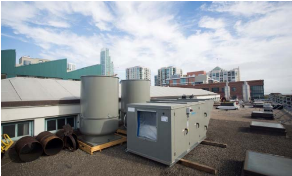
Pumping Station 1, new ventilation equipment with new engine exhausts in background
