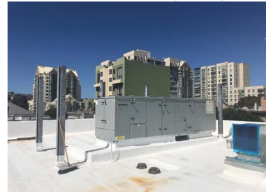
FS 5 – ERV Units Installed at Roof
