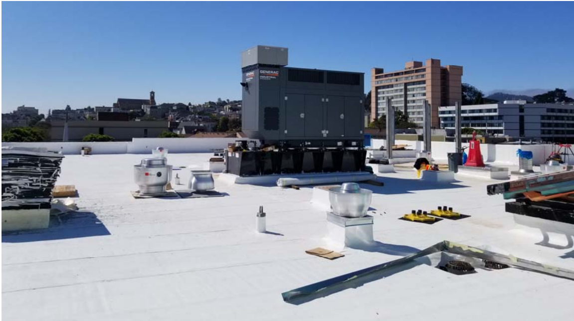
Emergency Generator, ERV Units, and Exhaust Fans Set at Main Roof (September 7, 2018)
