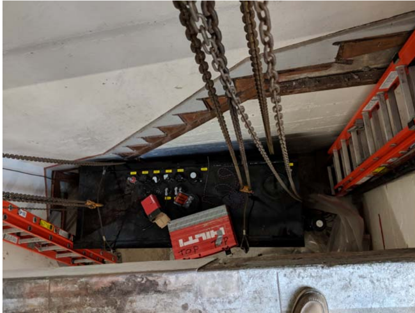
Back-up generator and fuel tank being lowered to basement level via hoist system.
