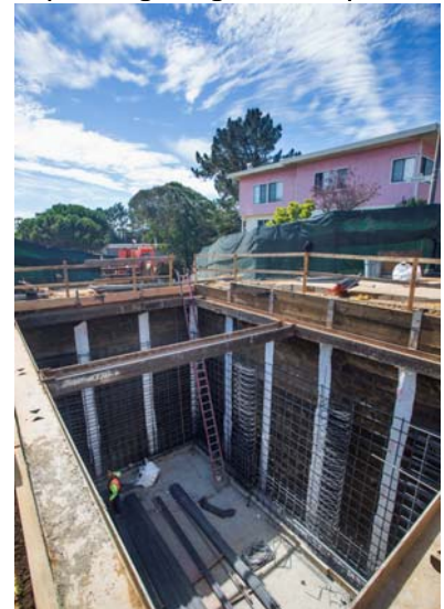
Amber Drive & Duncan Street Cistern
