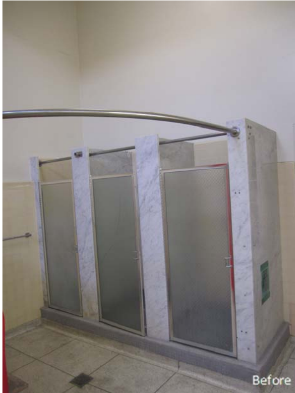
7432A Showers – Package 3 Station 38
