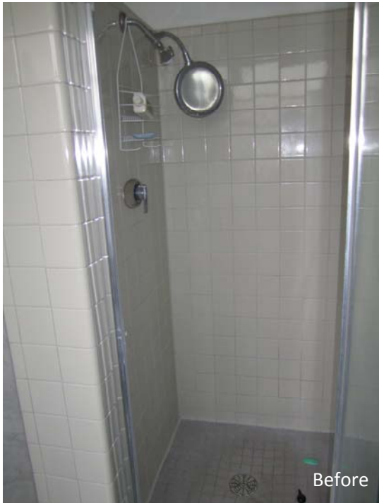
7432A Showers – Package 3 Station 41
